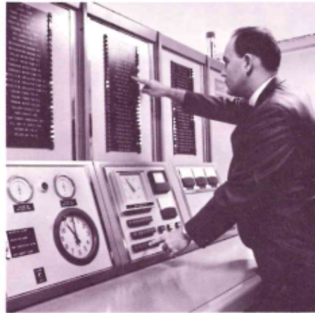
The maze of lights and buttons may look bewildering, but this Robertshaw control console helps the General Office building engineer maintain a comfortable environment inside, regardless of rain or snow outside. Andy Lane, Robertshaw project engineer, makes final tests.
